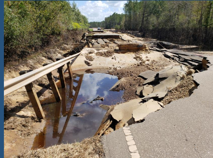
Flooding on NC Highway 210 at Moore's Creek from Hurricane Florence (2018)
